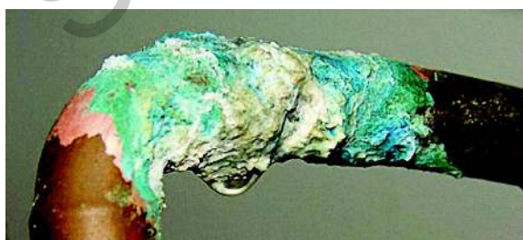
fig-18: Corrosion of copper
